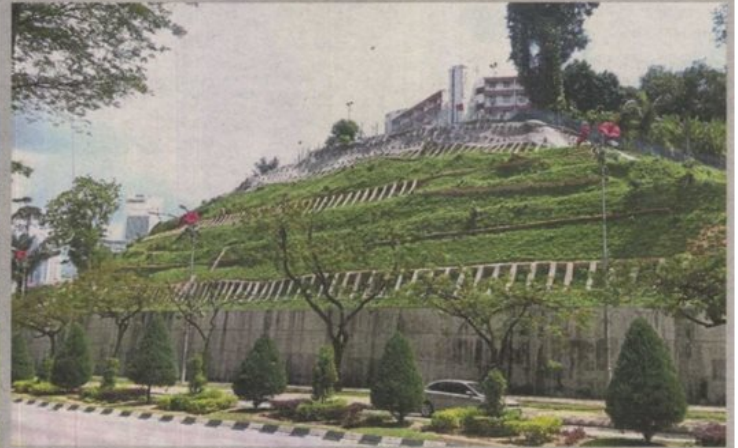
Completed slope strengthening works along Jalan Parlimen in Kuala Lumpur by Kuala Lumpur City Hall.
