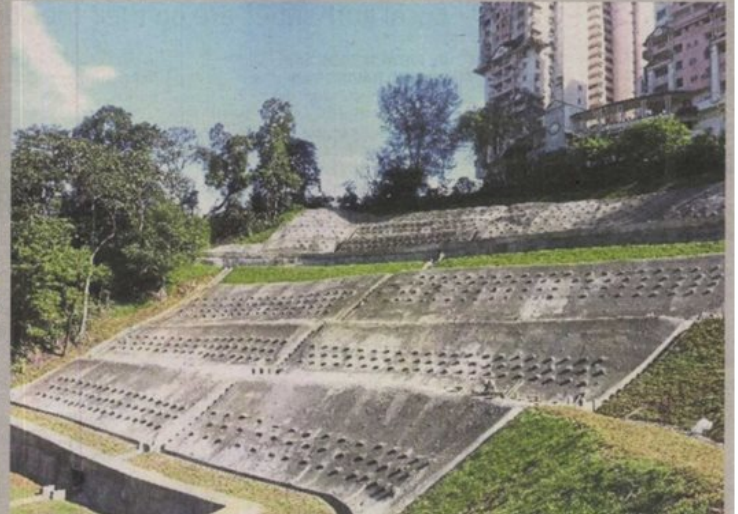
The Ampang Jaya Municipal Council completed the slope stabilisation works in Taman Bukit Utama, Bukit Antarabangsa in 2016.
